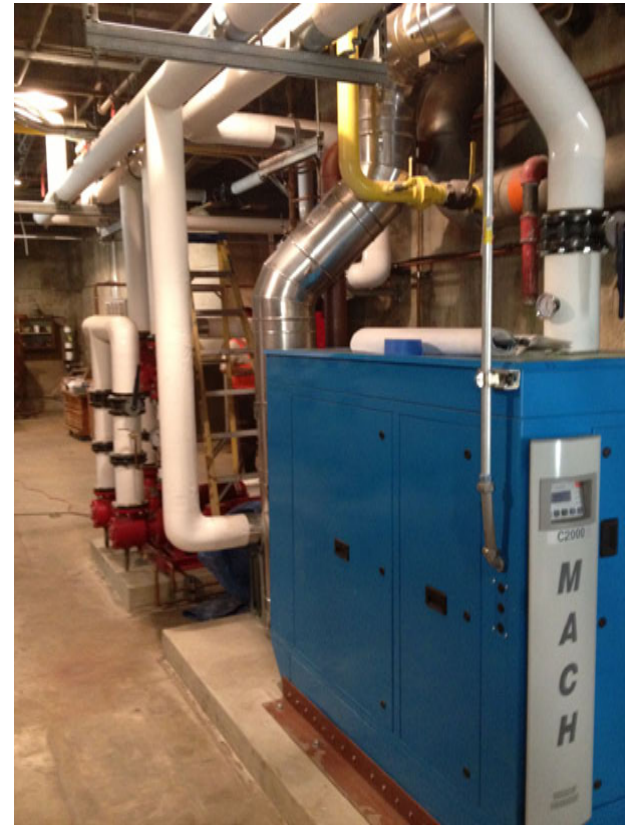
Millikan HS Boilers
