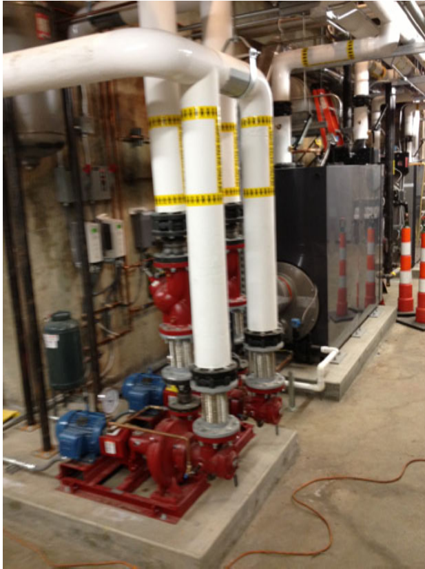
Lakewood HS Boilers
