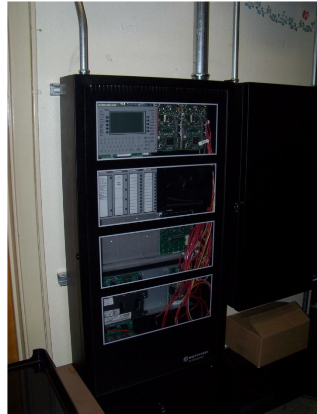
Lee ES – Fire Alarm Panel
