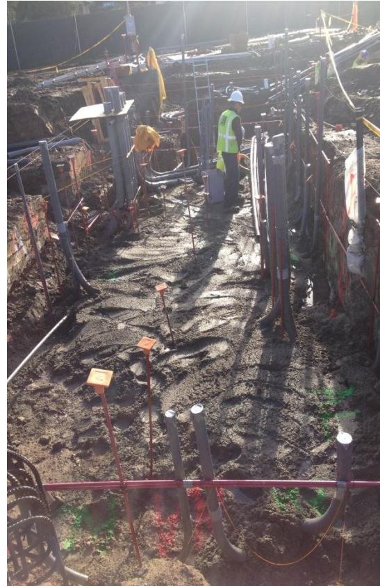
Main Electrical Room Slurry
