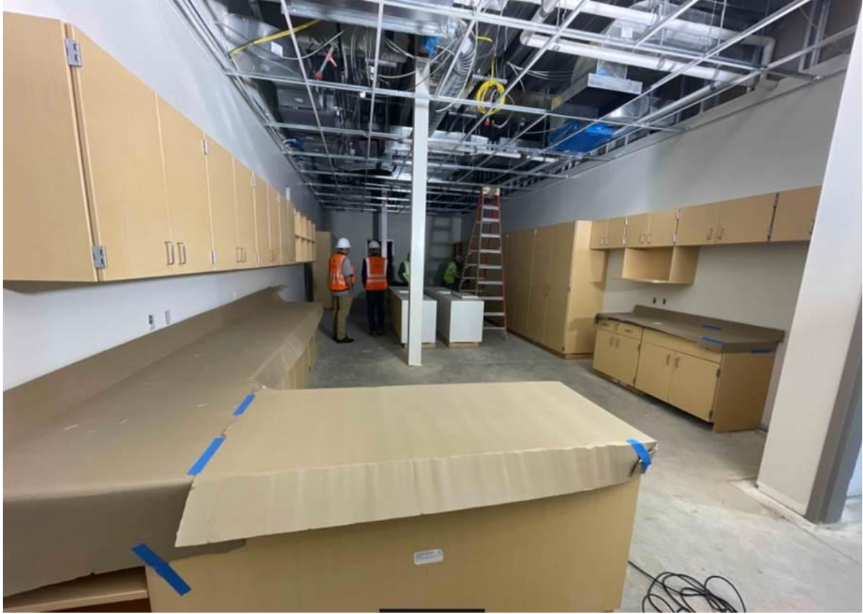
Cabinet installation in the Academic Wing's administrative office area
