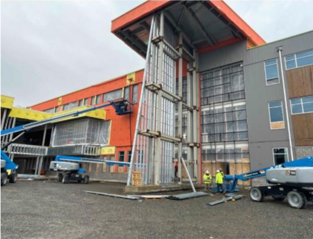
Crews working on the framing and window system at the main entryway
