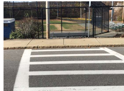
Missing ramp on Fulton St.
