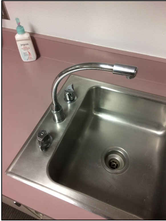
Sample HHH122216-P-CF-06: 19 µg/L initial lead concentration. Fixture style above is identified producing elevated lead concentrations.
