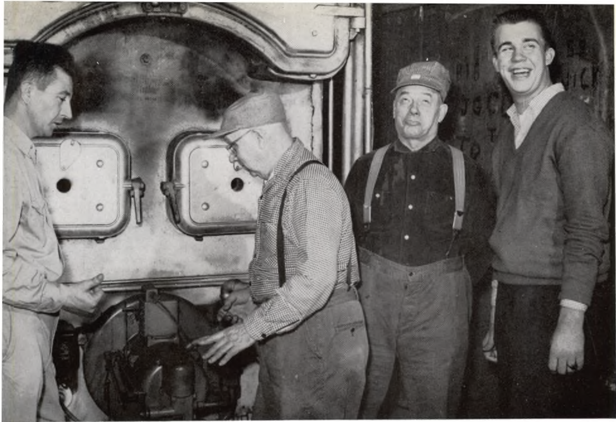
Mr. Drenth shows Mr. Meers how to operate the boiler while Mr. Dykstra and Ken Deters look on.
