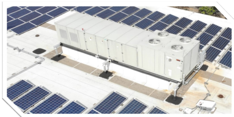
Air Conditioning Upgrade Project – Phase I (North Stratfield Elementary School, Osborn Hill Elementary School & Fairfield Woods Middle School)
