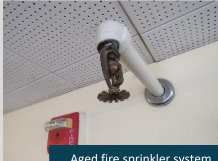
Aged fire sprinkler system
