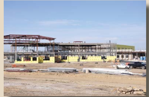
Construction is approximately 50 percent complete on Wilson Middle School, on schedule to open this August.
