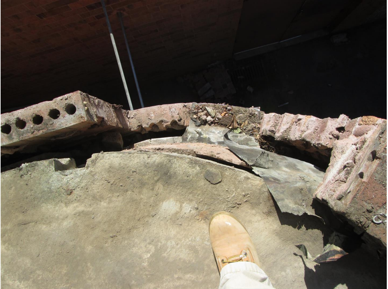
Photo C – throughwall flashings found at the plan south east corner of the building.
