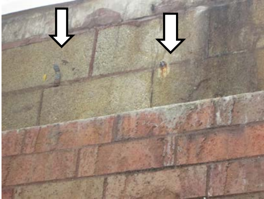
Photo E – corrugated ties in place with rust near the limits of the concrete masonry unit wall
