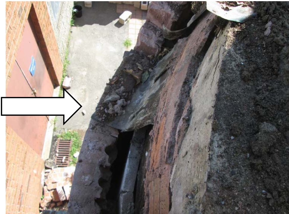
Photo I – fabric coated copper throughwall flashing found approximately six courses below the concrete roof deck elevation.
