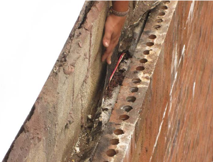
Photo Q – rusted conduit exposing the electrical wires within the cavity wall.
