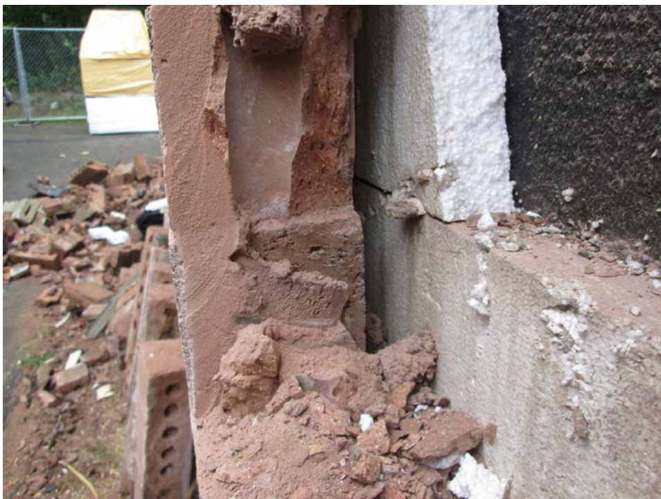
Photo M – South elevation; location one – west side of test cut; the eyehooks of the adjustable ties were in place in the backup wall, but the pintle was not installed. Note that the mortar joint is continuous in this location, and not disturbed, indicating that the wall anchor was not in place.
