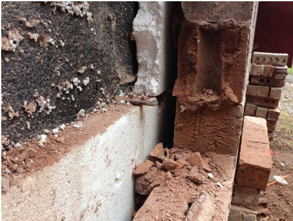
Photo K – South elevation; location one – east side of test cut; the eyehooks of the adjustable ties were in place in the backup wall, but the pintle was not installed. Note that the mortar joint is continuous in this location, and not disturbed, indicating that the wall anchor was not in place.
