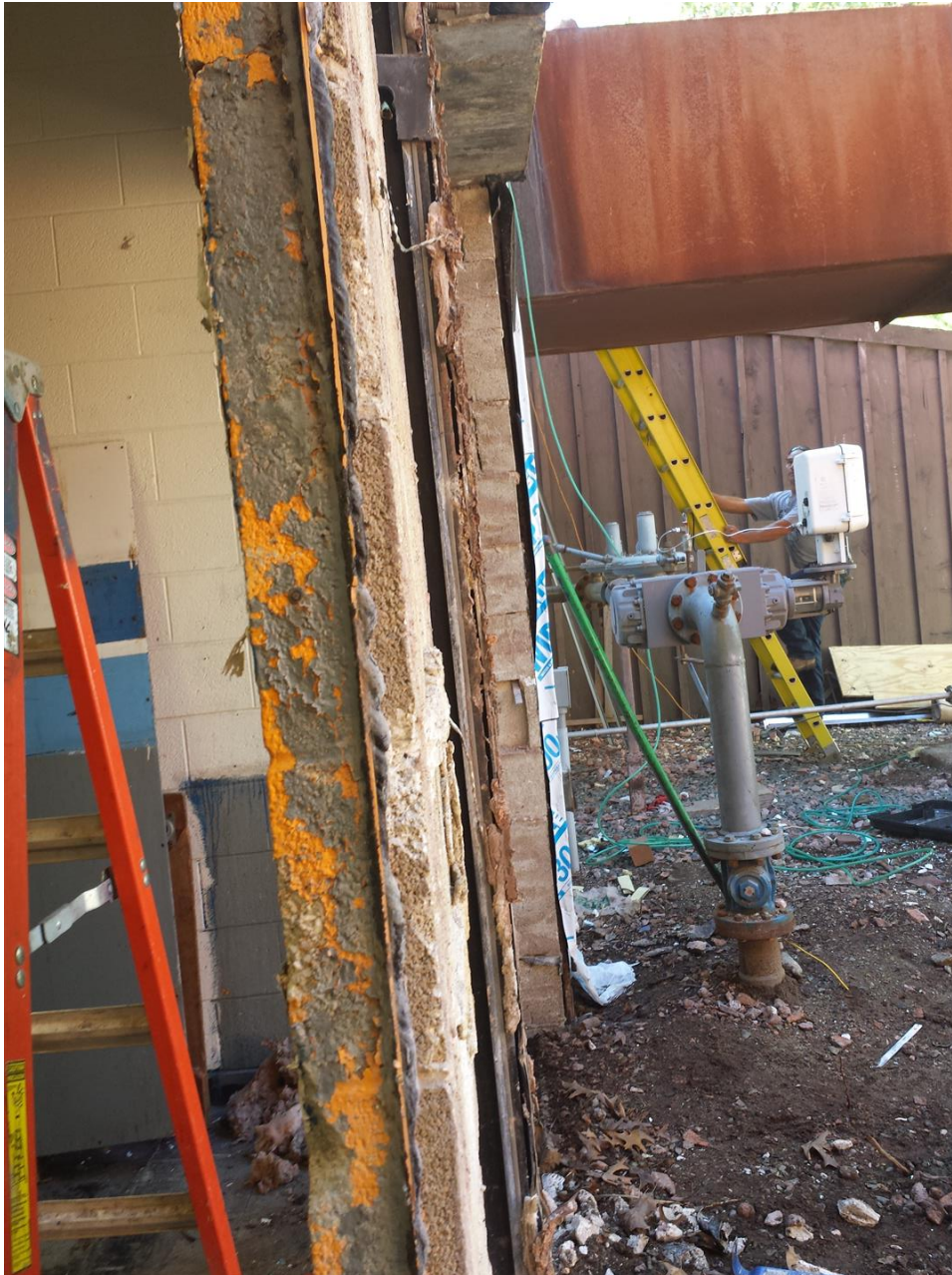
Photo E – existing column leans inward, towards the building.
