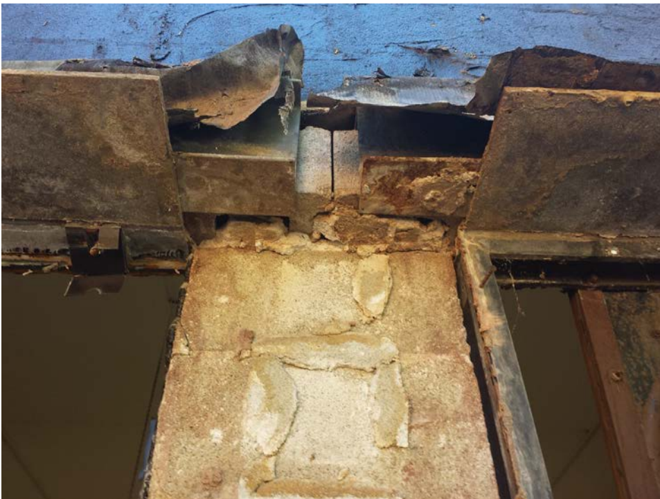
Photo D – lintels are not continuous, and rest on the CMU
