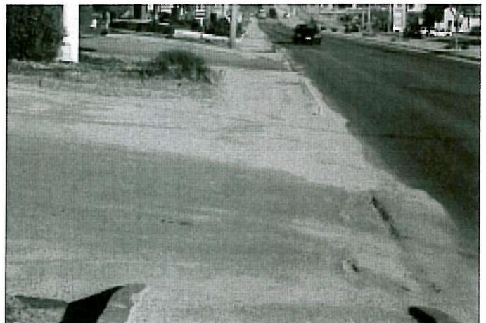
The predominance of curb cuts along this roadway creates an unsafe/uninviting environment for the pedestrian.
