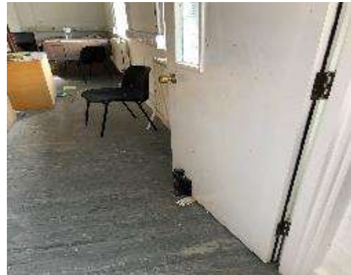
Science and technology fire doors wedged open
