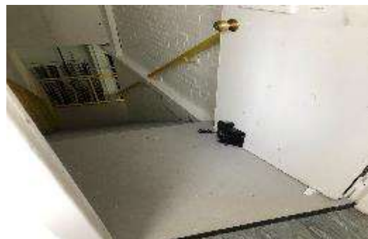
Science and technology fire doors wedged open
