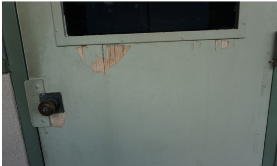
Doors and door hardware in need of replacing.
