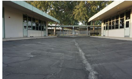
Flooding issues between buildings.
