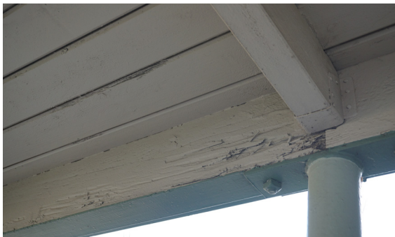
Building fascia boards need attention.
