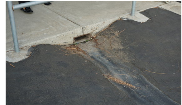
Drainage issues around campus.
