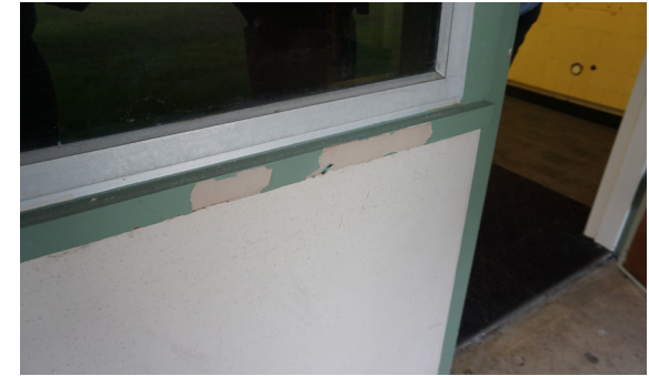
Window trim in need of replacing.
