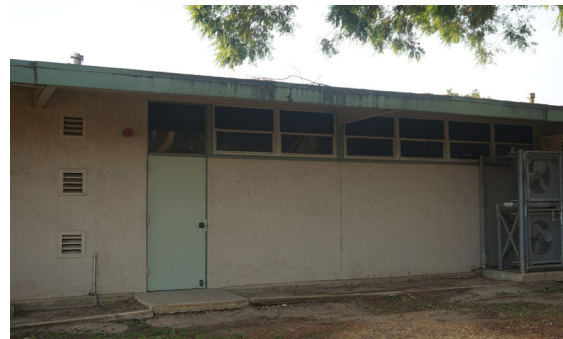
Building exteriors need attention.
