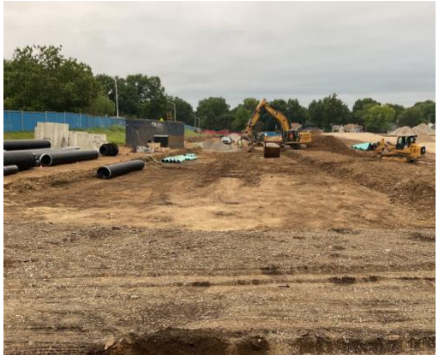
Sanitary Main Piping
