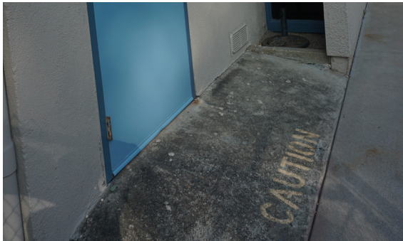
ADA issues in circulation areas between buildings.
