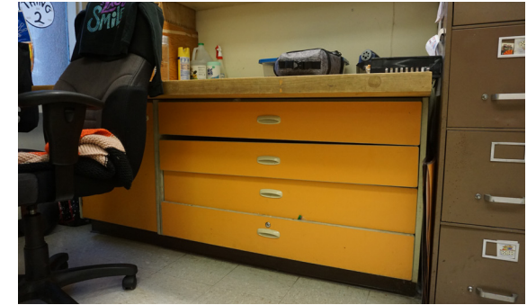
Typical casework in classrooms need replacing.
