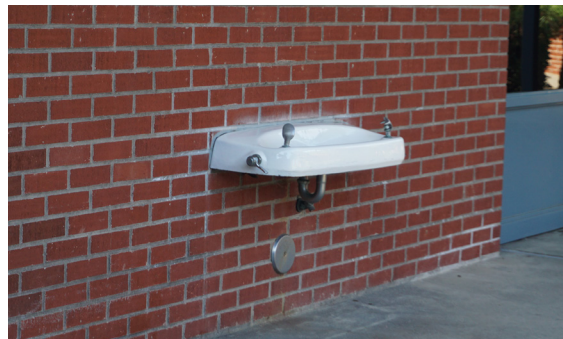
Typical water fountain.
