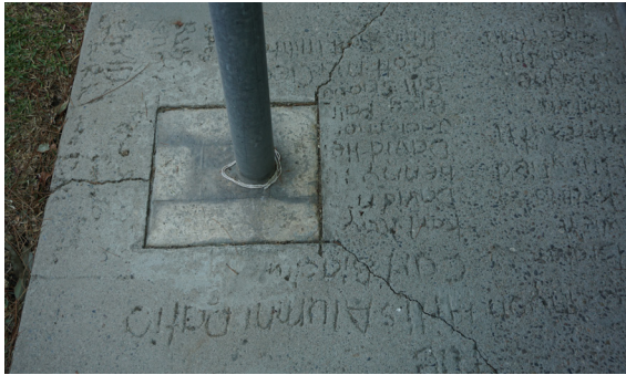
Cracked concrete under lunch shelter.
