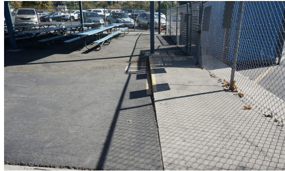
Drainage issues near lunch shelter.
