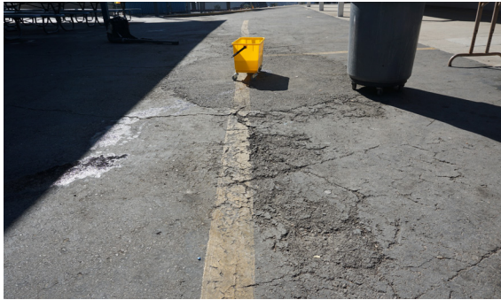
Lunch shelter's ground condition needs attention.
