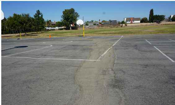
Flooding issues on hardcourts.
