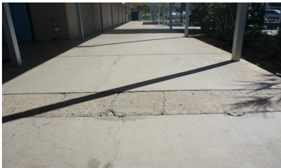
Cracked concrete pads on main walkways.
