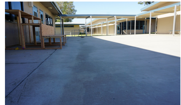
Flooding issues between classrooms.
