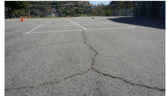
Cracking on hardcourts.
