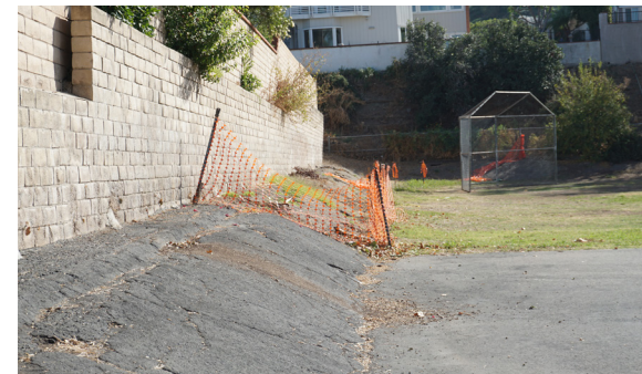
Safety hazard with damaged slope adjacent to hardcourts.
