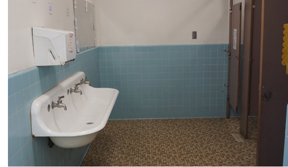
Restroom fixtures in need of an update.
