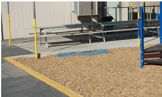
Play structure ground in need of replacement.
