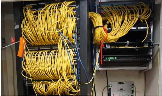
In need of proper IDF storage.
