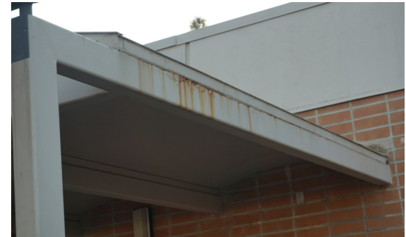
Building exterior in need of attention.
