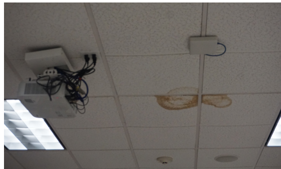
Classroom ceilings in need of attention.
