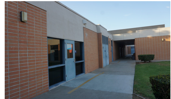
Classroom thresholds lack shade and weather protection.
