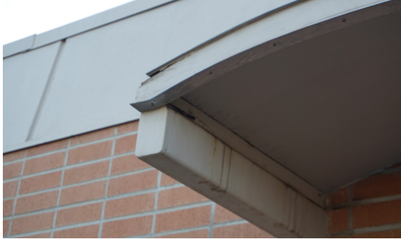
Building awnings in need of attention.
