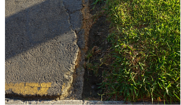
Cracking ground condition.
