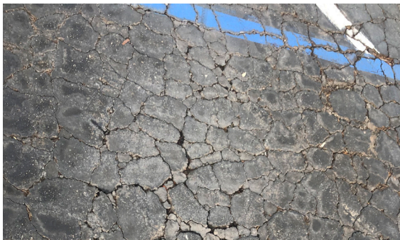
Cracked parking surface.
