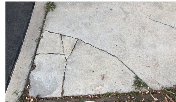
Cracked concrete pads on playground.
