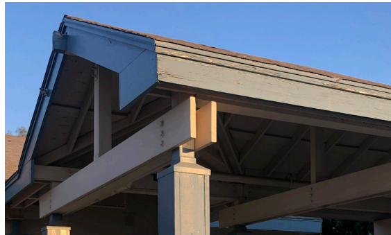
Fascia boards in need of an update.
