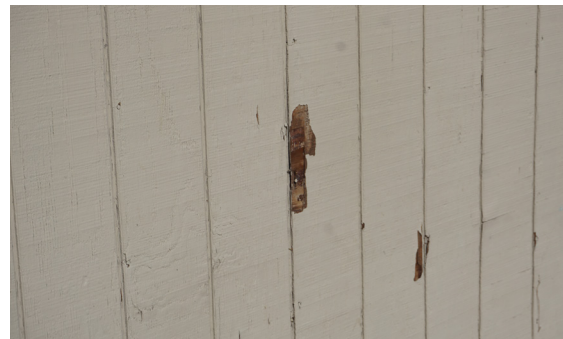
Aged and damaged portable condition.
