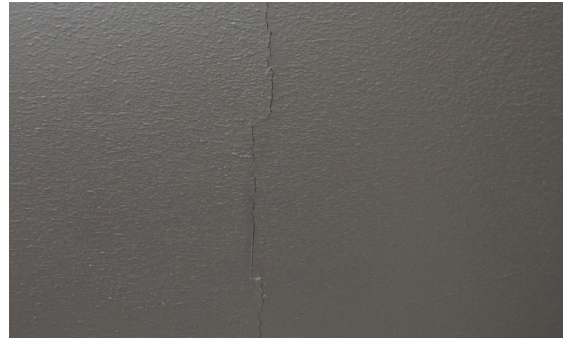
Cracked paint on interior walls.
