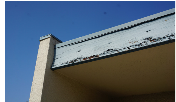
Fascia boards need attention.
