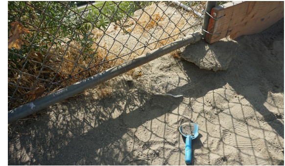
Safety issue with fencing gaps overlooking cliff.
