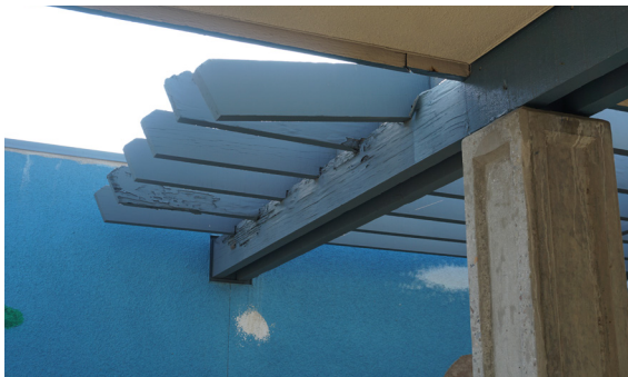
Wooden\ shade structures need attention.
