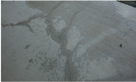
Cracking and flooding issues around campus.
