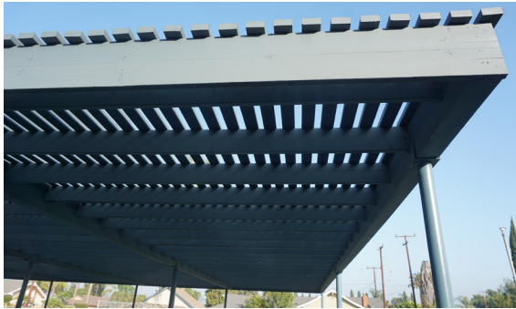
Wood-slat lunch shelter needs replacing.
