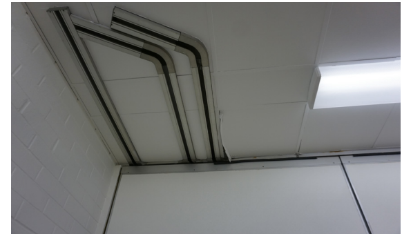
Inoperable foldable partitions need replacing.
