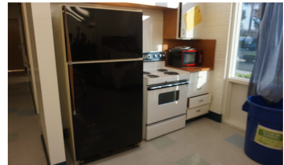
Outdated fixtures in teacher break room need replacing.
