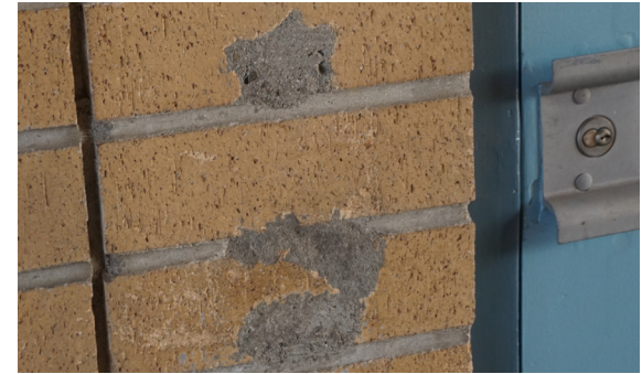
Building exteriors need refurbishing.
