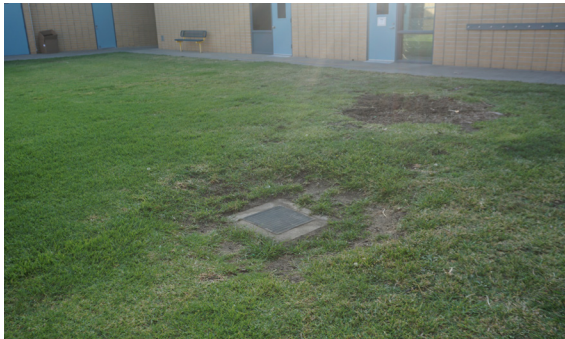
Drainage issues cause landscape damage.
