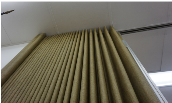
Outdated operable partition in teacher workroom needs replacing.
