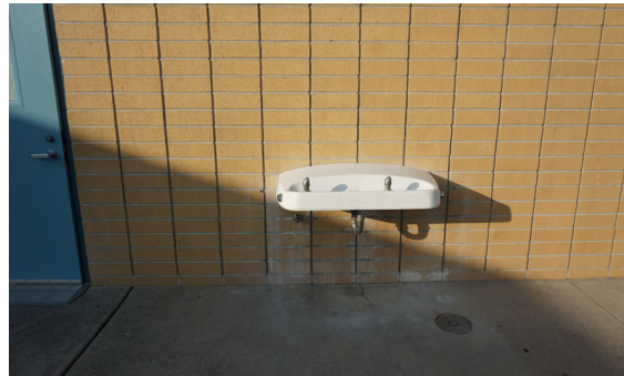
Outdated water fountains need replacing.
