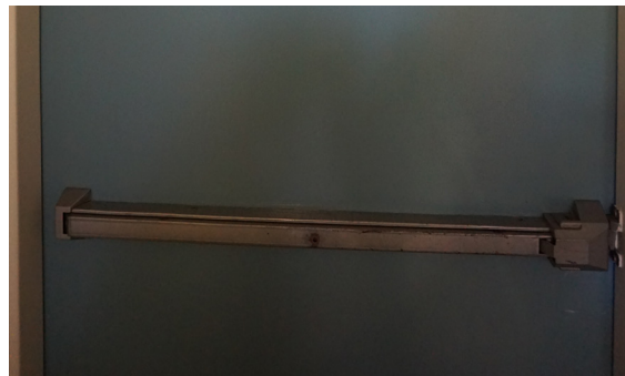
Outdated panic hardware needs replacing.
