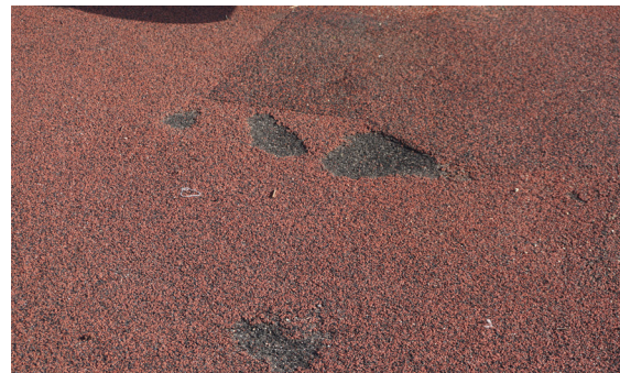
Play structure surface damaged, needs replacing.
