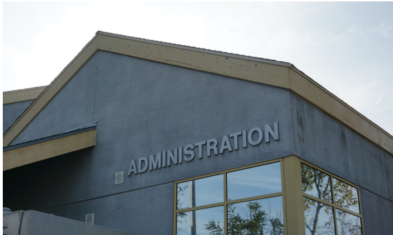
Administration building needs new paint.
