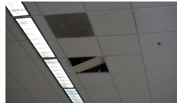
Broken ceiling tiles in Multi-Purpose room.
