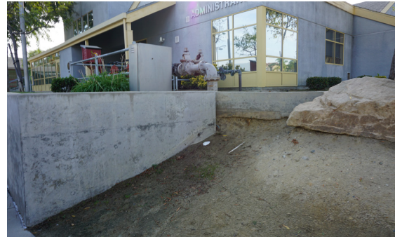
Flooding issues at the front of campus.
