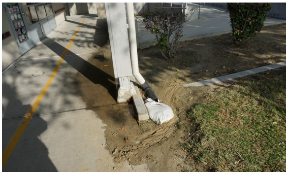
Drainage issues between classrooms.
