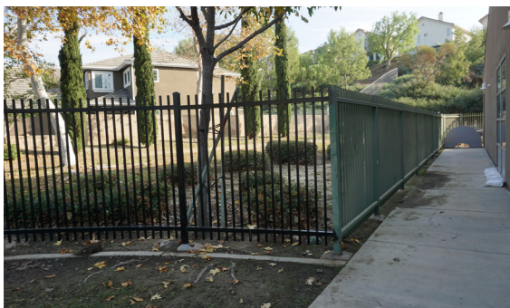
Fencing is not continuous.
