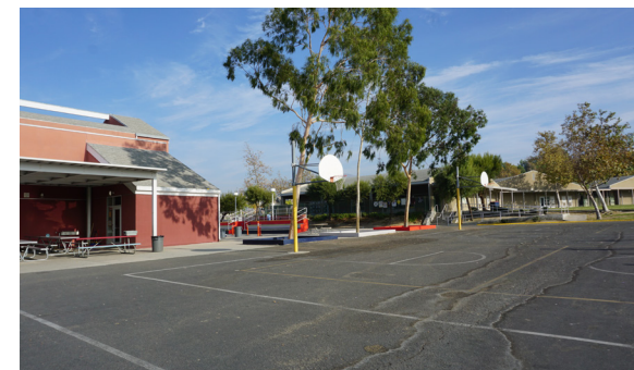
Drainage and flooding issues on hardcourts.
