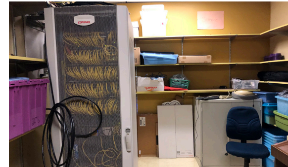
Inappropriate storing of IDF.
