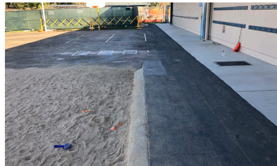
Sand in kinder play area needs to be replaced.
