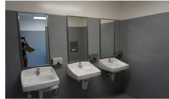
Typical restroom fixture.
