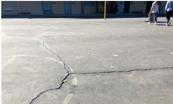
Cracking across hardcourts.
