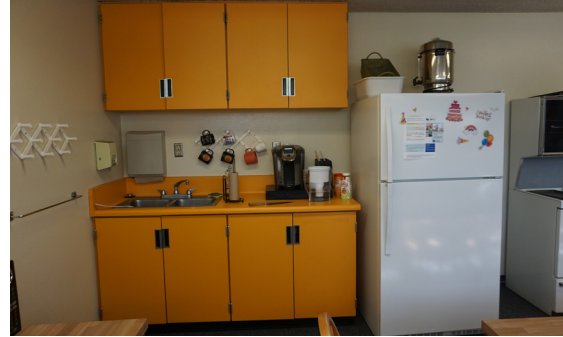
Outdated casework in teacher workroom.
