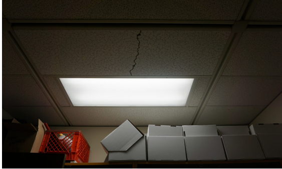
Cracked ceiling tiles.
