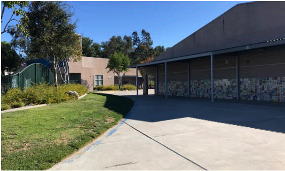
Patchy grass areas and lifting concrete pads.
