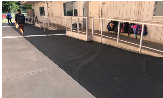
Cracking and flooding near portables.
