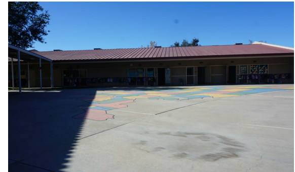
Puddling in quad area.
