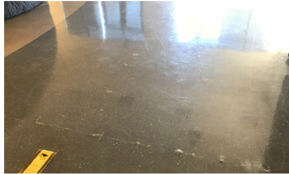
Damaged floor in MPR.
