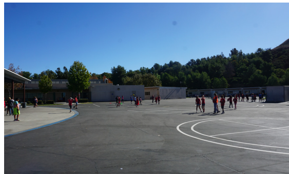
Cracked asphalt in hardcourt area.
