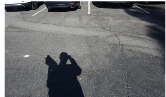
Flooding and cracking in parking lot.
