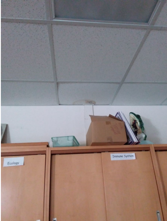
133 Stained Ceiling Tiles
