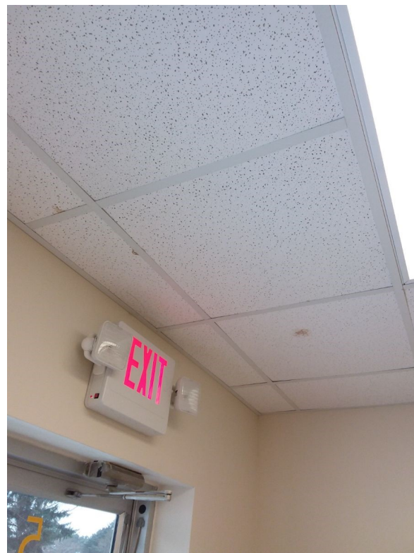
119 Stained Ceiling Tiles
