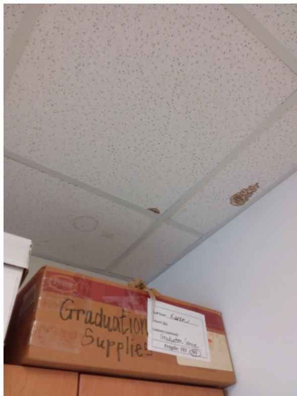
119 Stained Ceiling Tiles
