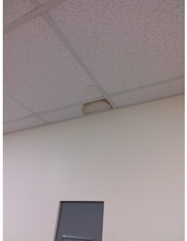
114 Stained Ceiling Tiles
