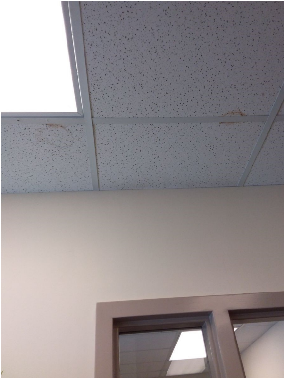
MAIN RECEPTION Stained Ceiling Tiles
