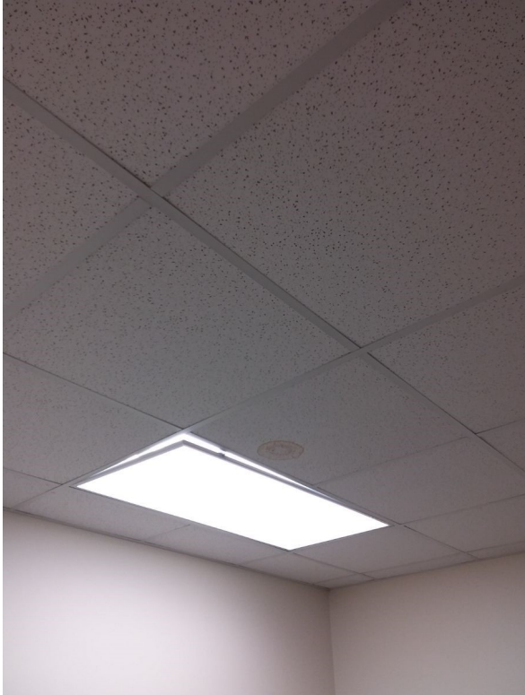
112 Stained Ceiling Tiles
