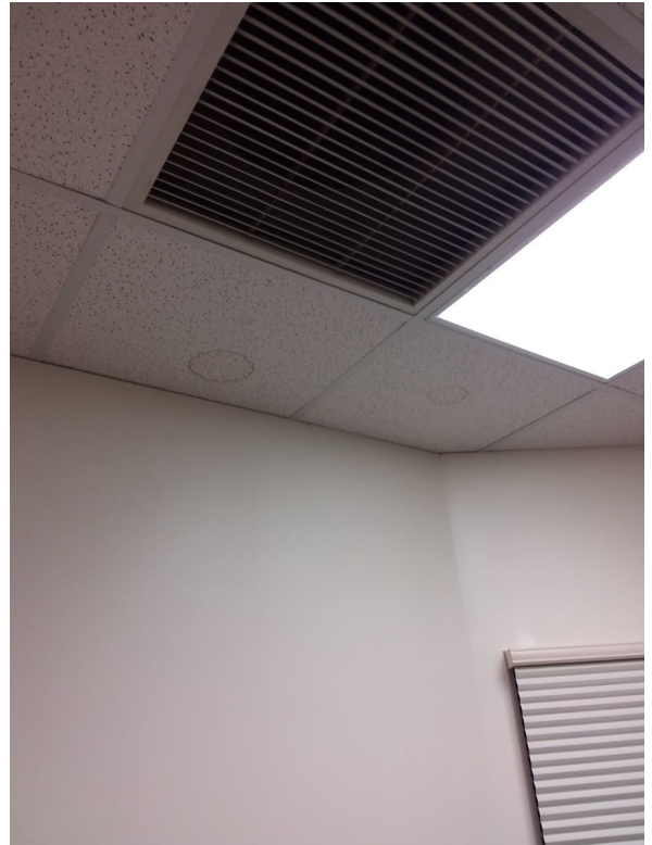
125 Stained Ceiling Tiles
