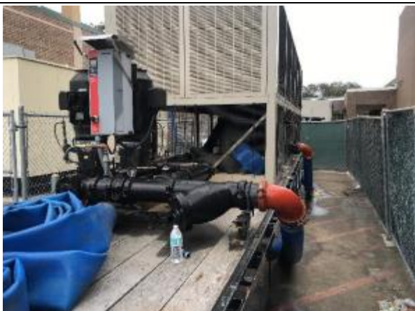
Temporary chillers have been connected to the building.
