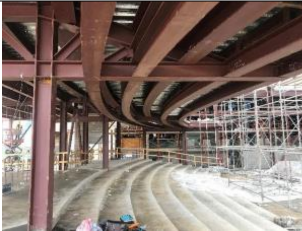
Ductwork support straps are being hung from the steel deck above the foyer.
