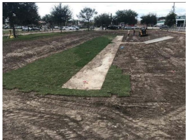
Sod is being placed in the South Detention Pond Basin. North Pond to follow.
