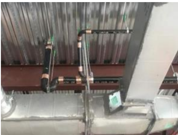
Cast iron drain lines are being installed below the mech. mezzanine deck. Mechanical duct joints are being sealed.
