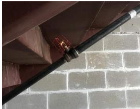
Fire sprinkler lines have been installed under the stair to the mezzanine
