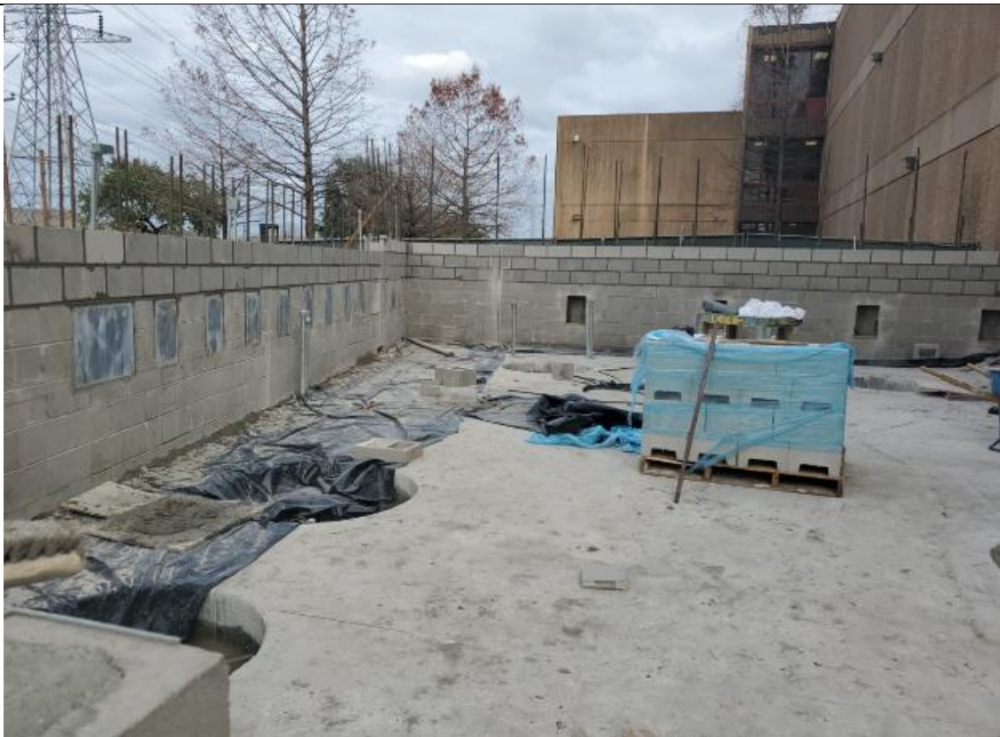
Inside photo of the chiller yard.
