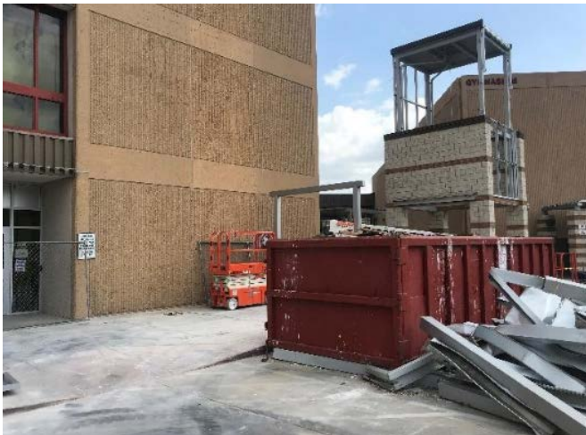
Portions of the aluminum walkway cover, along with the sidewalk, has been demolished.
