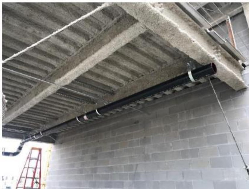
Cast iron drain lines and fireproofing are being installed at Phase I building addition.
