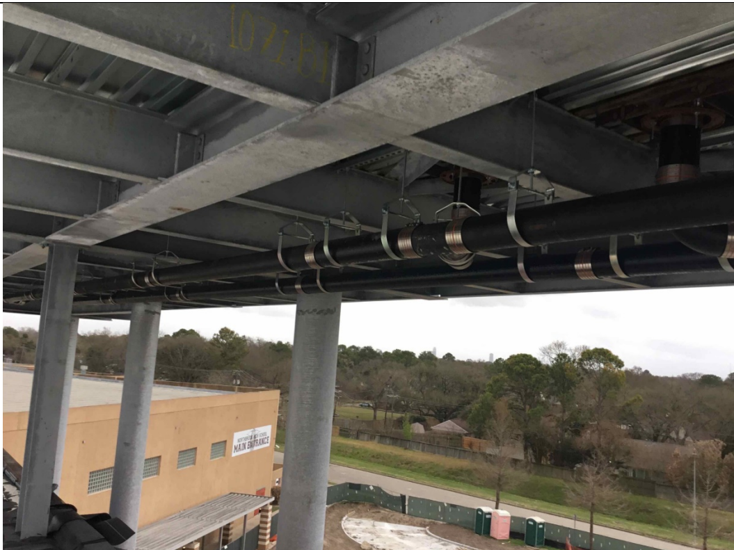
Additional image of the cast iron drainage at the High Bay Canopy.
