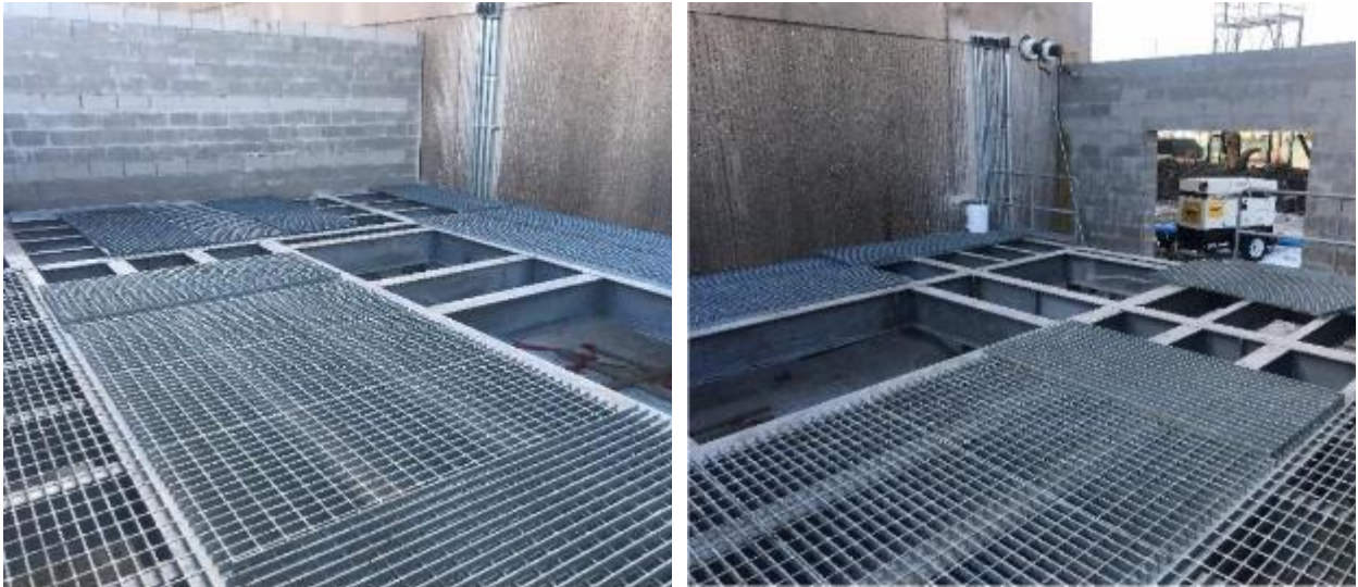
CMU masonry work around the chiller yard perimeter has been completed. Galvanized platform structure and grate placement is on-going
