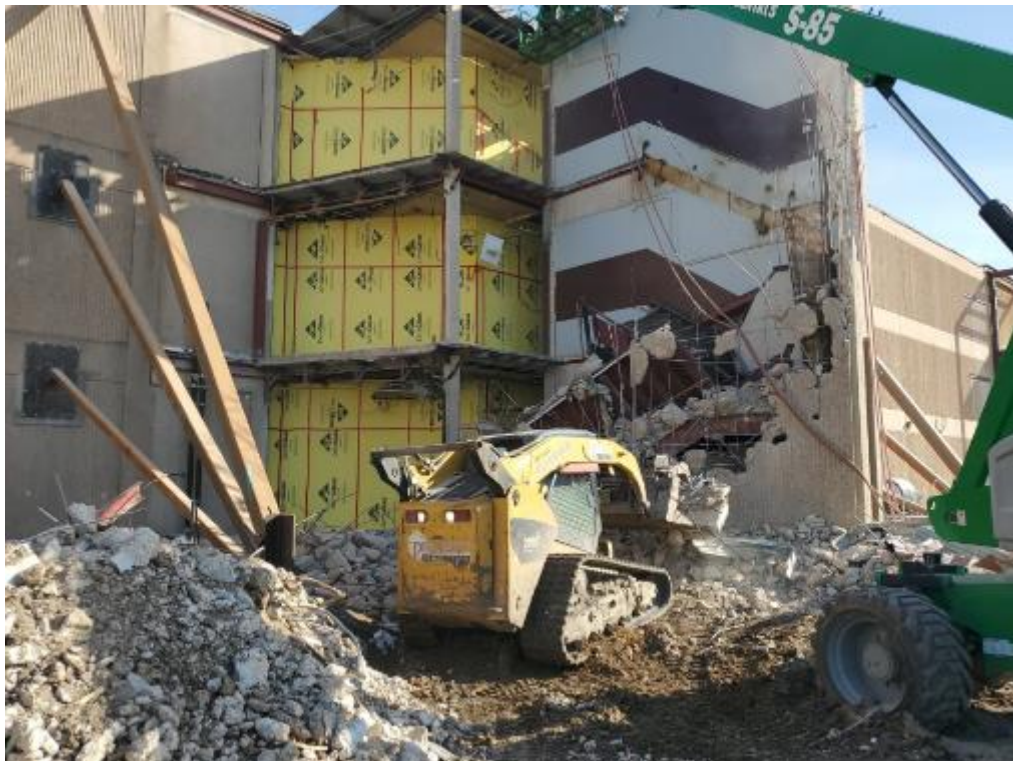
Portions of the existing stairwell have been demolished. The existing interior corridor has been protected with metal studs and exterior sheathing panels
