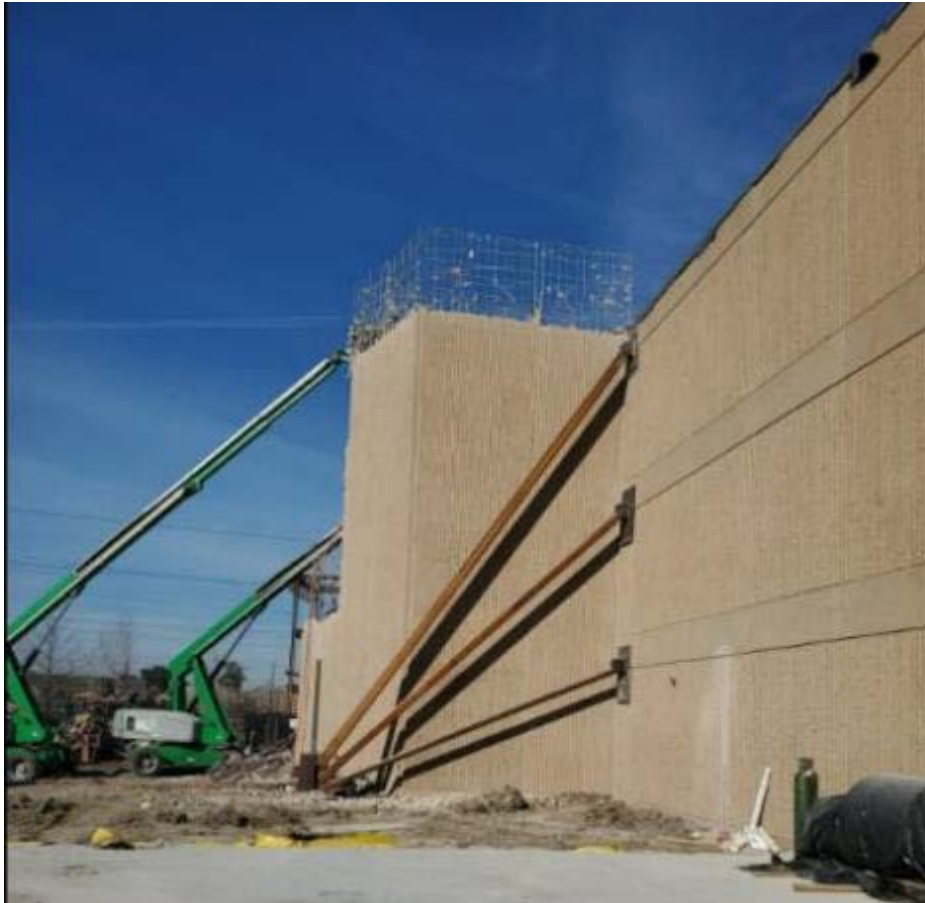
The steel bracing to support the existing tilt-wall has been installed and anchored.
