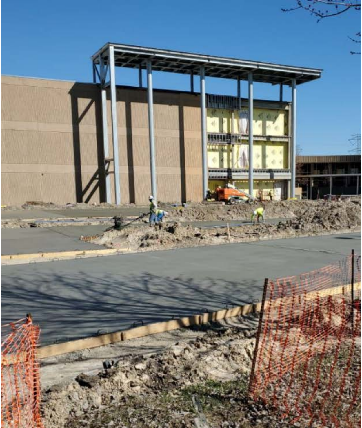
Concrete has been installed at the main entry and new south drive.
