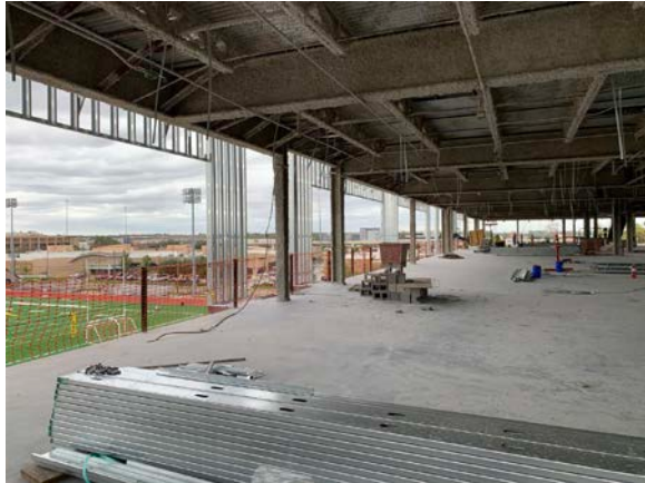
Exterior metal studs (CFMF)
