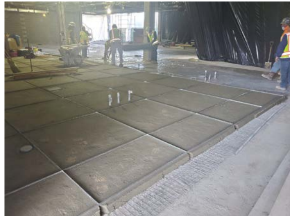
Area NA1 terrazzo at servery
