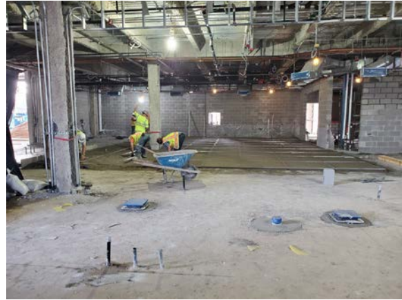
Area NA1 terrazzo at servery
