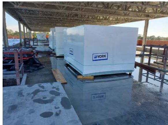
Mechanical enclosure with equipment
