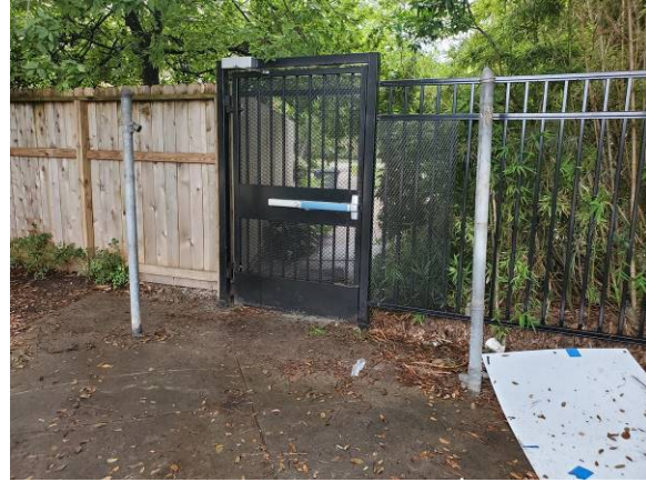
Completed secure gates at neighborhood
