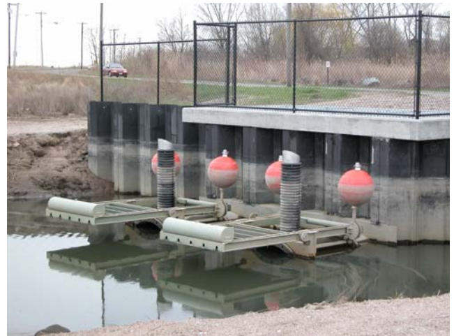
Self-regulating tide gates (SRTs) increase tidal flow without causing upstream flooding. Photo courtesy of Roger Wolfe.
