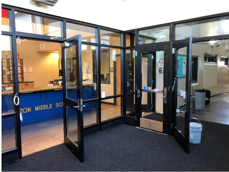
New storefront doors and glass panels are being installed at Horizon MS and is near completion.
