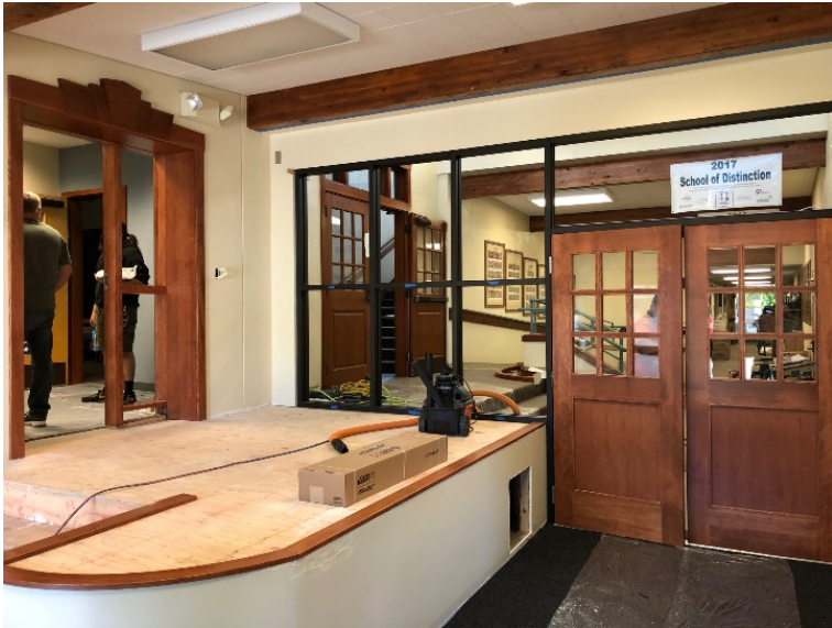
Central Elementary secured entry is taking great shape with new doors and hardware going in.
