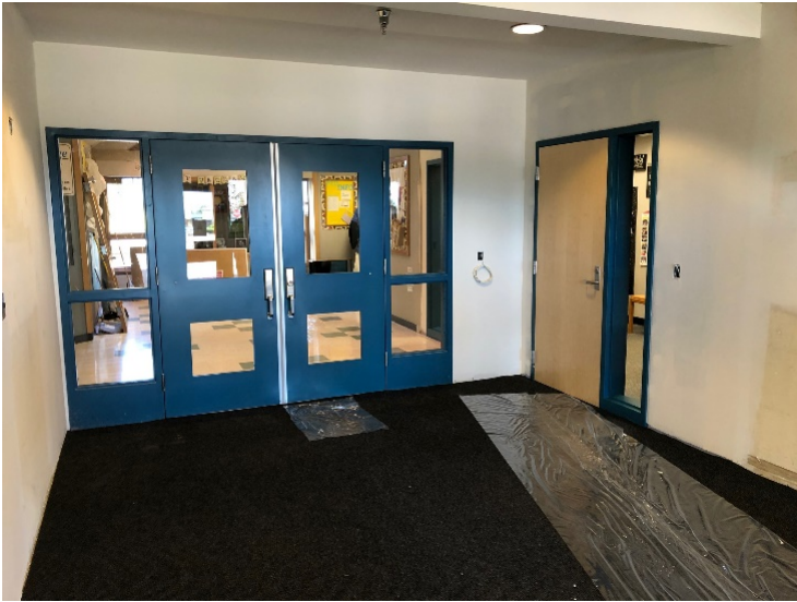
The Eagleridge hollow metal frame doors have been relocated for the secured entry.
