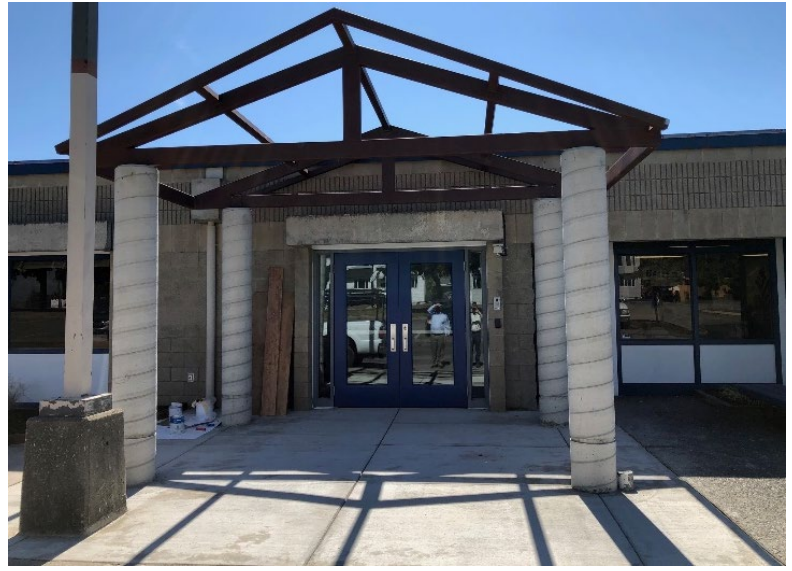
Concrete is complete at the new secured entry at Skyline Elementary with trusses in place.
