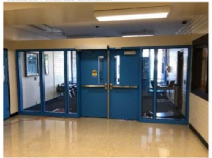
Vista MS: The new entry vestibule that directs all visitors into the office.
