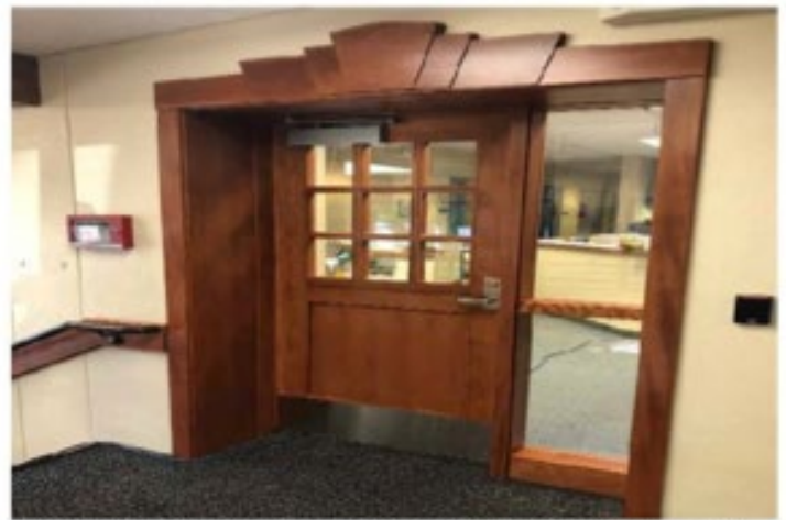
Central ES: Visitors will need to be buzzed in and enter the office through this new door from the vestibule.
