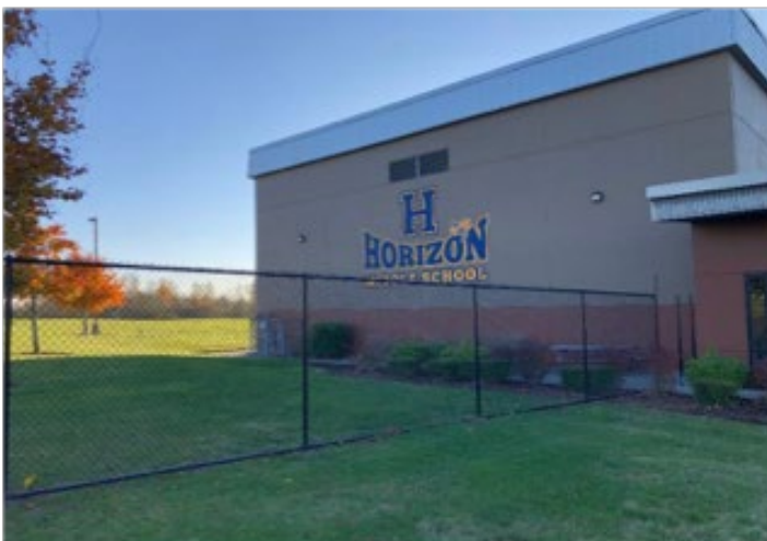
A new 7 foot high fence and new gates are being installed to secure both sides of Horizon Middle School.
