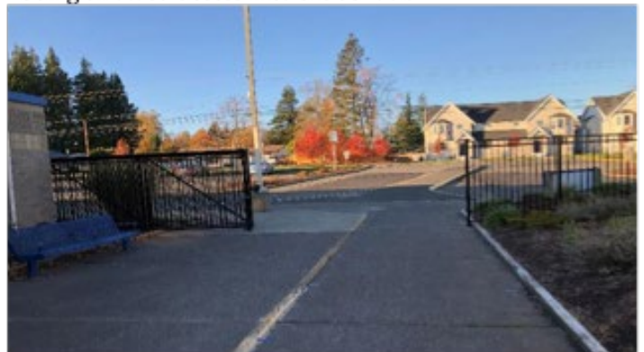
Skyline Elementary perimeter fencing and gate installation is complete. Gate hardware is being installed that will be locked daily once school starts to provide additional security.
