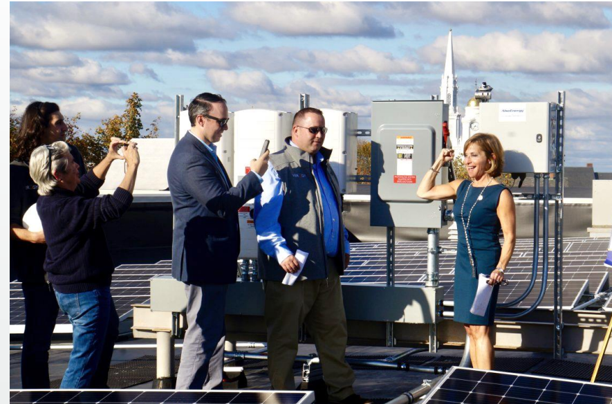
Mayor Cantor and Council Members Sweeney and Kerrigan activate Town Hall's solar array, October 2019.
