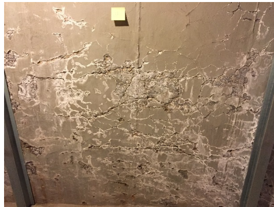
(c) map cracking
