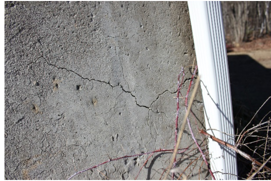
(c) map cracking
