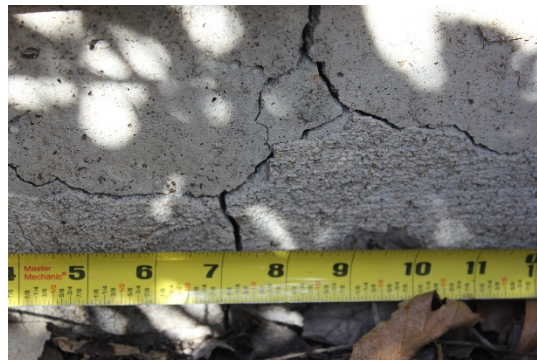
(c) wide crack opening
