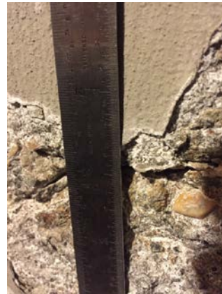
d) crack opening (>4mm)
