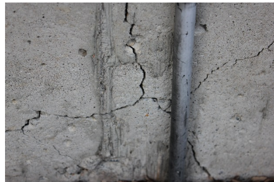
(b) map cracking
