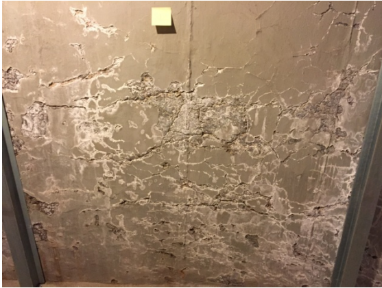
a) map cracking
