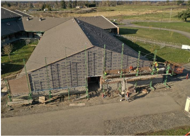
Waterproofing membrane is installed and masonry work continues on the south side.
