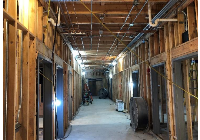
A view down the interior hallway showing door frames installed, plumbing and electrical work.
