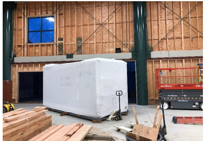
The large air handler/heater has arrived and will be installed in a 2 nd floor mechanical room.
