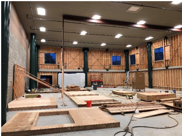
The new gym center beam has been installed and walls for the storage & mechanical room are ready.
