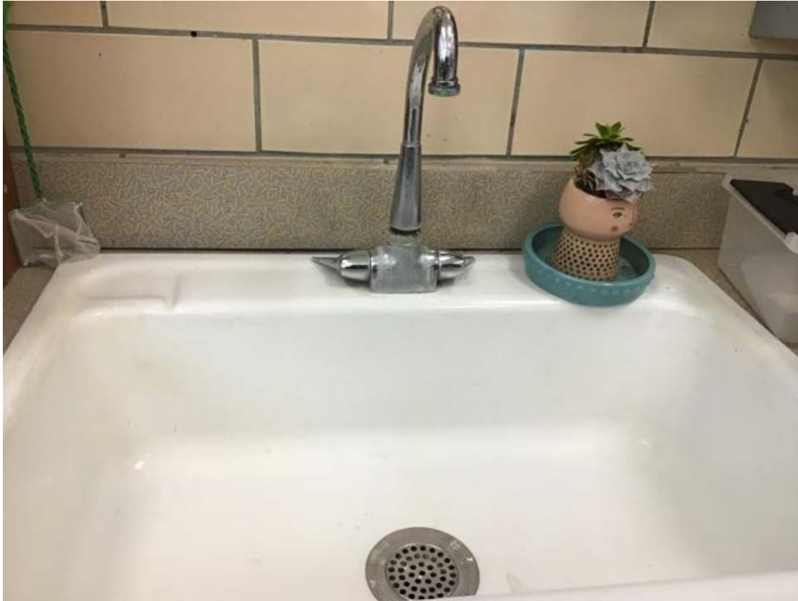
Jefferson-03: Room 116, Faucet
