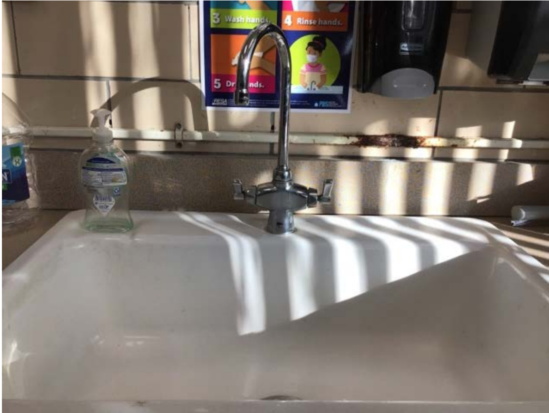
Jefferson-04: Room 118, Faucet
