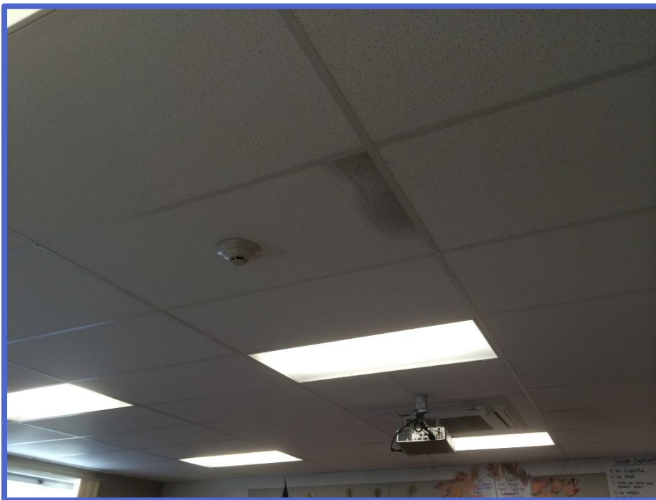
Figure 3: Leaking refrigerant can be seen saturating ceiling tiles in a classroom at Dorsa Elementary
