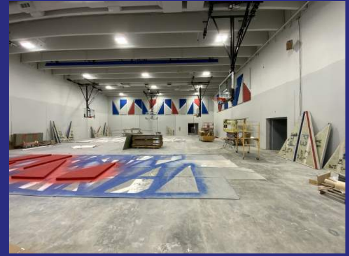
Gym - Equipment & Panels
