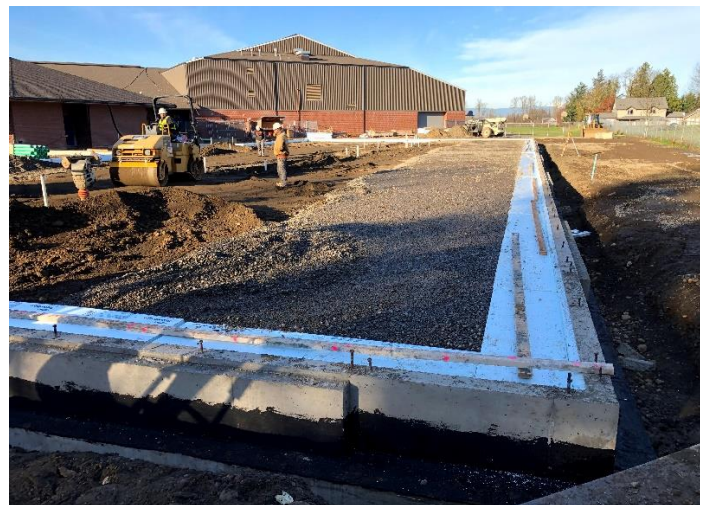
Perimeter foundation insulation and the capillary break are both shown in this photo.
