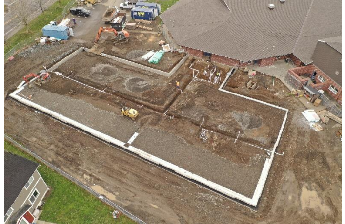
Drain rock is being placed on the east side of the new classroom addition.
