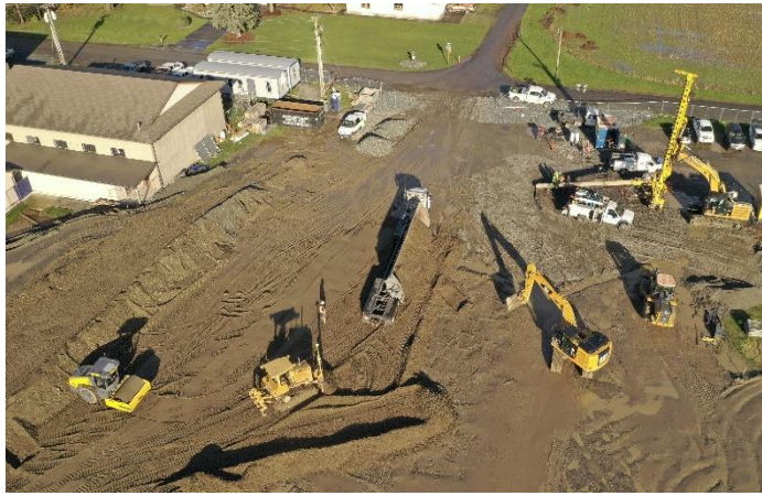
This drone aerial photo was taken on 11-19-2020 showing a large dump truck dropping gravel.
