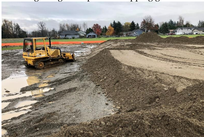
The east pad now has approx. 4 feet of pre-load gravel placed and compacted.
