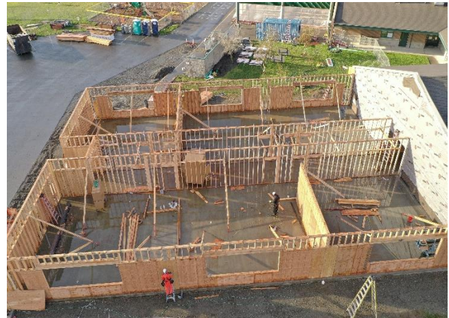
A closer look showing the 6 classrooms & shear walls. Bathroom walls still to be framed.
