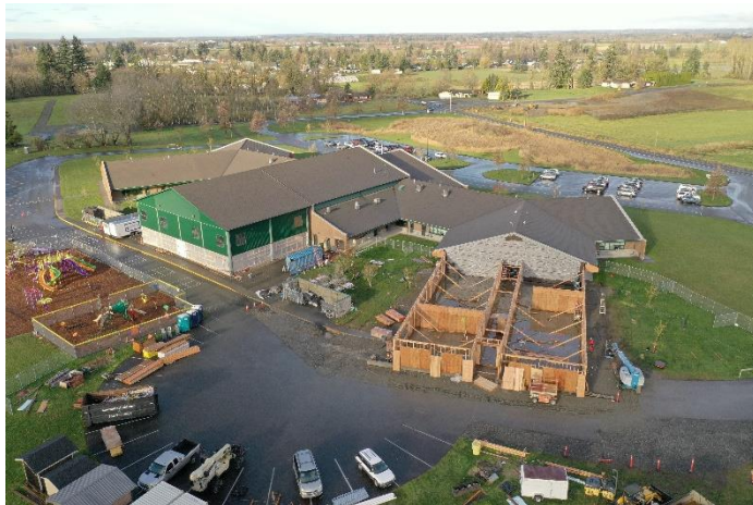
These drone aerial photos were taken November 19 and show the main walls all framed up.
