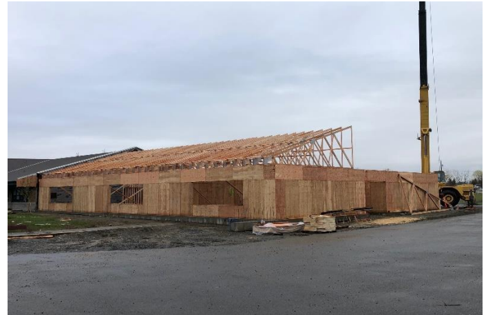
Trusses went up on Nov 23. This image captures the first half of trusses placed on the west side.
