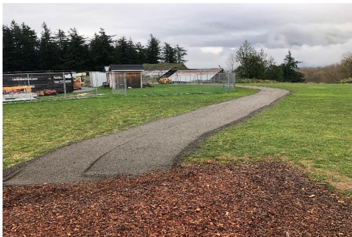
A gravel walk path was installed today to provide students with clean access around the construction area to the playground.
